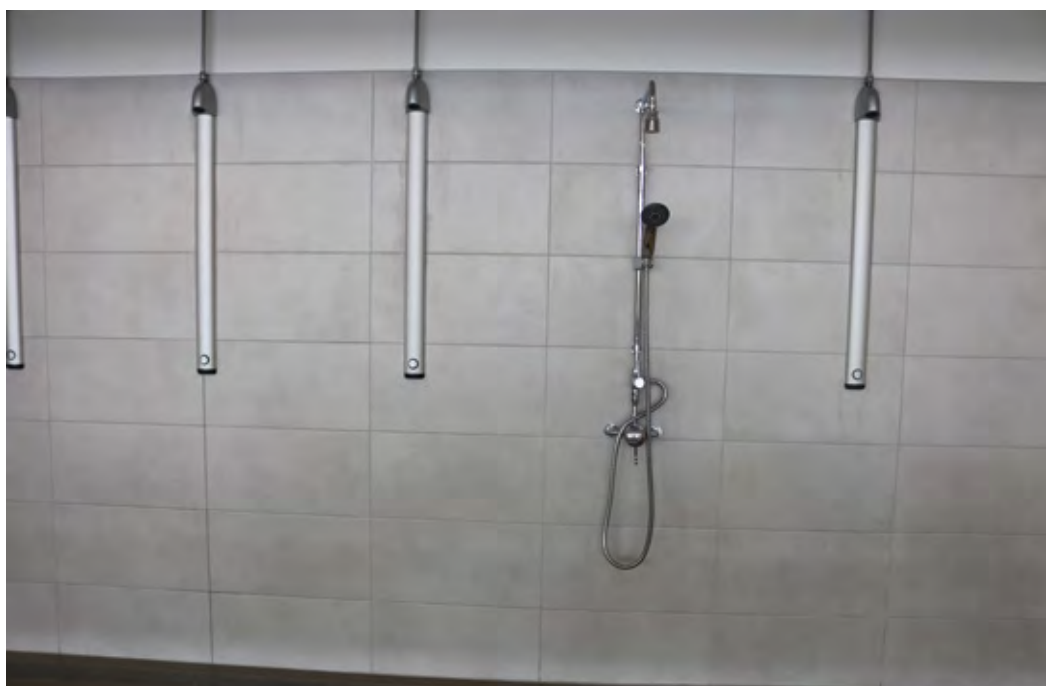
Accessible shower provision within row of standard use pre-swim showers (South Lake Leisure Centre)
