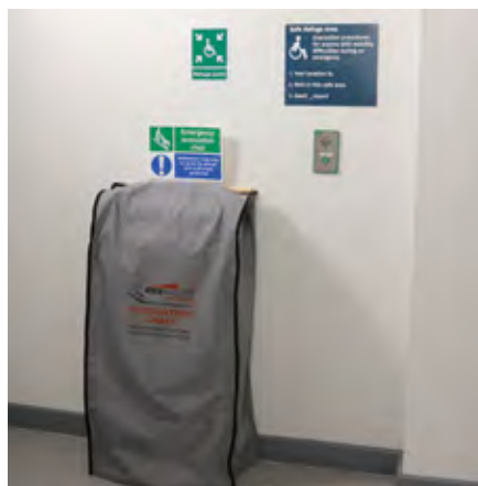
Refuge area and evacuation chair (South Lake Leisure Centre)
